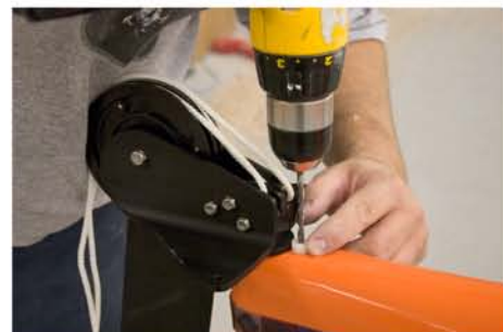
1.2-Place the plastic washer on the rudder; drill a hole with a 3/16 bit.
